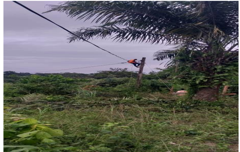
Electricity extension to Assin Kramokrom CHPS compound.
